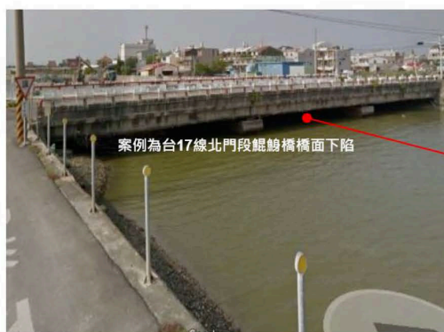
鯤鯨橋橋梁底座及橋墩長期浸在河中
