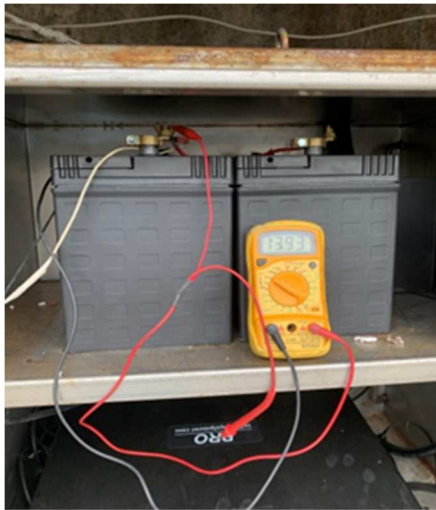
(a)岸上蓄電池組維護
