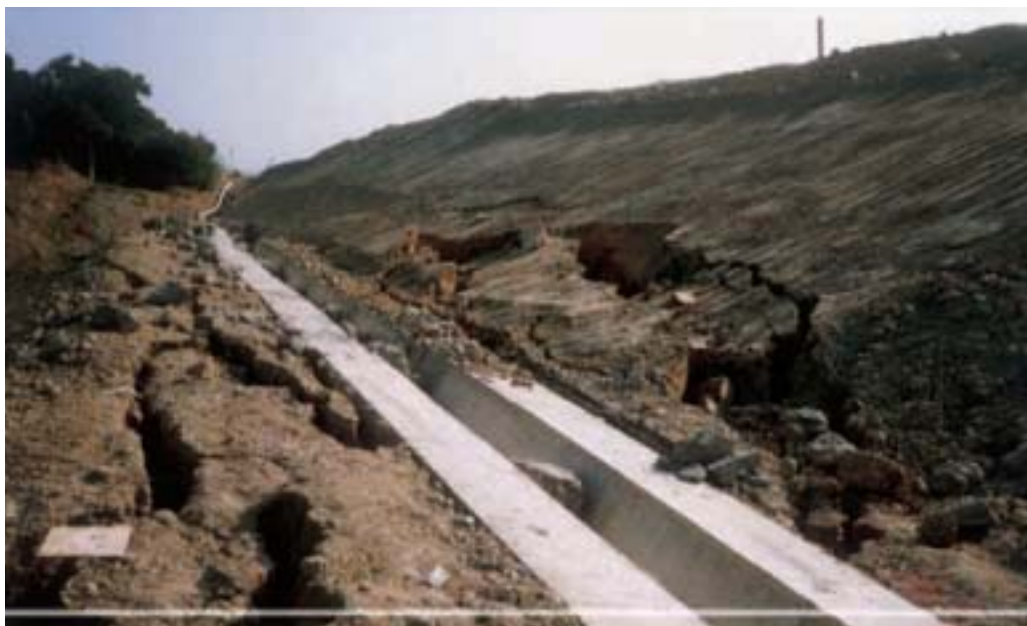
266k+830m邊坡坍塌坡趾隆起全貌
