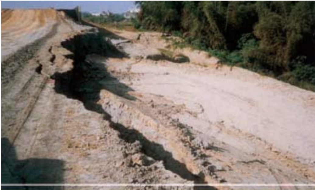
266k+830m邊坡坡頂坍塌全貌
