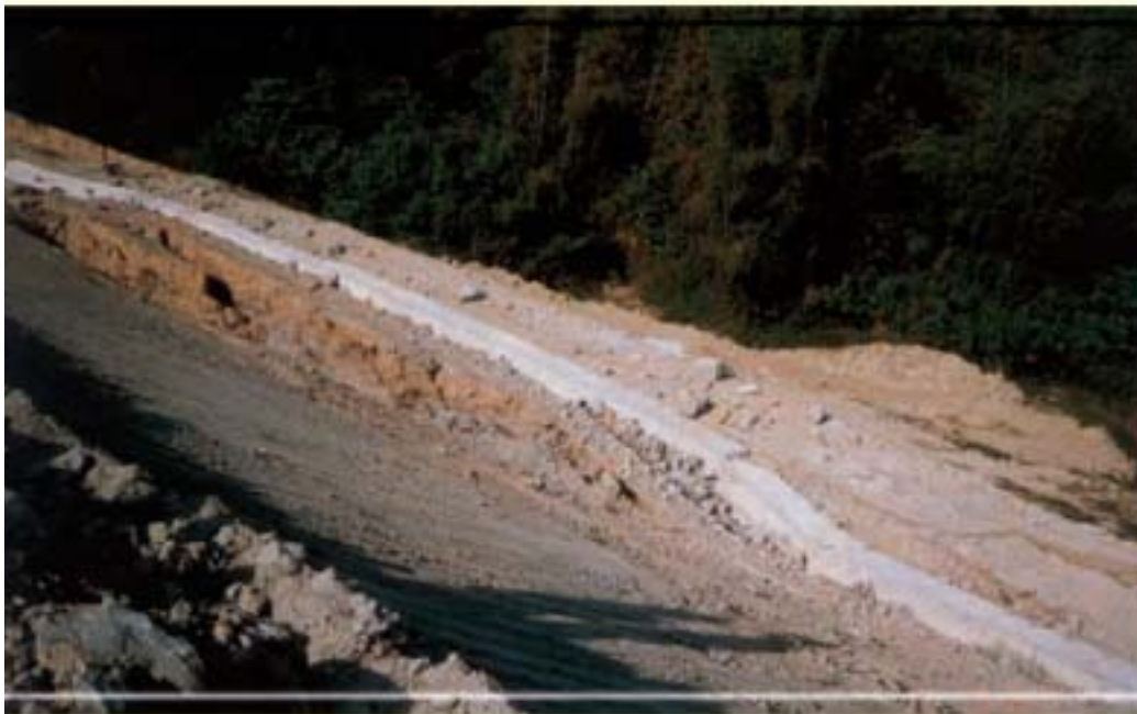
266k+830m邊坡坍塌坡趾隆起全貌
