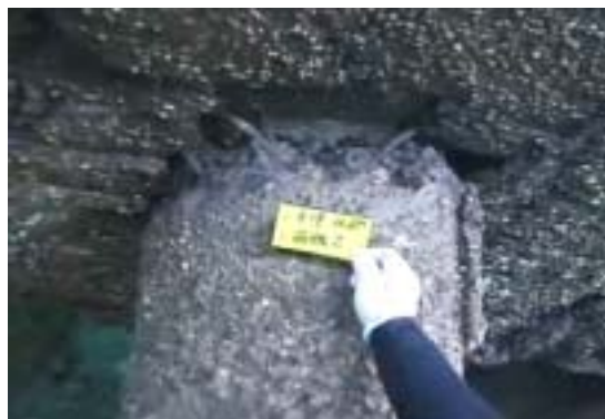
(2) 面版與樁頭交接處鋼筋外露
