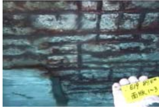
(2) 面版與樁頭交接處鋼筋外露 2
