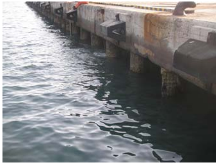
碼頭基樁與護舷材情形
