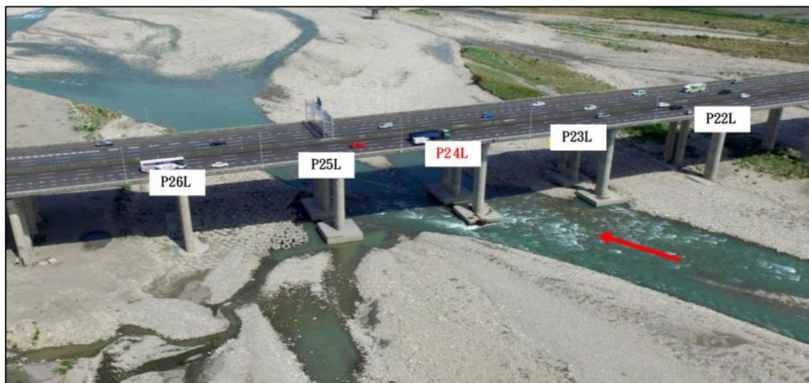
Figure 3: River conditions at the test bridge site (P24L) prior to the tribar armor + geotextile laying protection technique.
